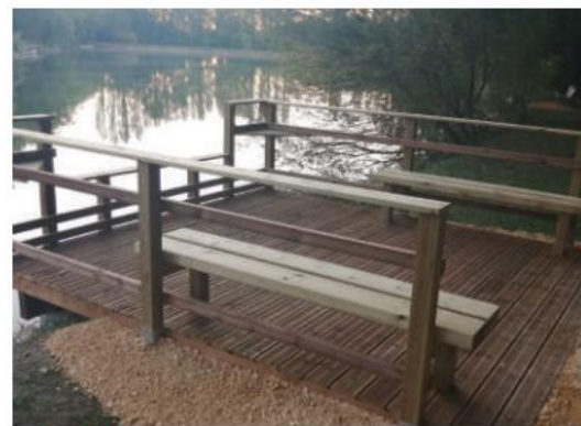
Fishing pontoon built by Technical Services as part of the "Family Journey" label © L. DAROT
